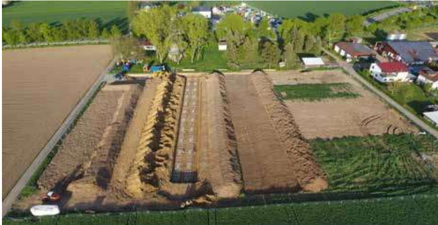
Fig. 9: Drone image geothermal heat collector
