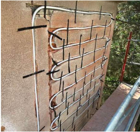
Fig. 17 'Sani60ies' project: Milling the pipes into the concrete blocks © Institute of Building Research & Innovation ZT GmbH
