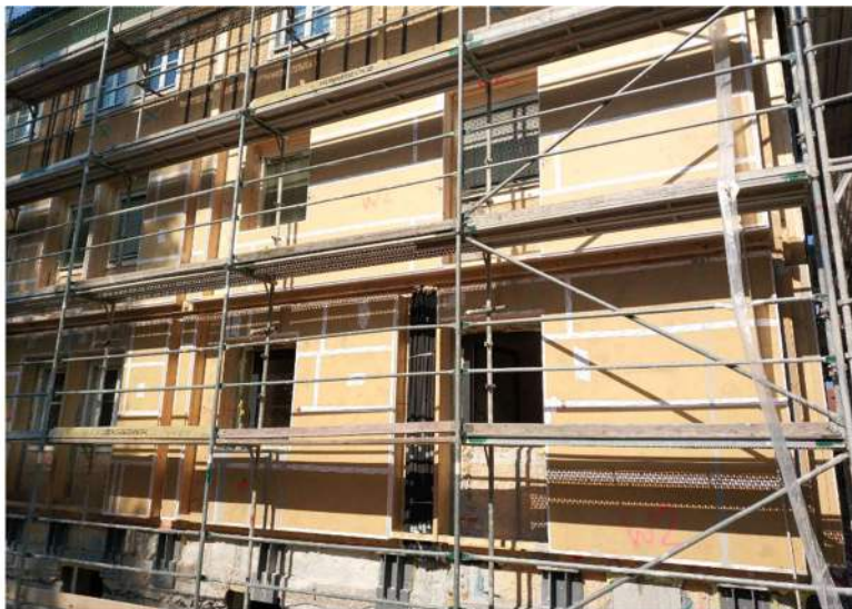
Fig. 14 ‘Wohnen findet Stadt’ Installation of the prefabricated façade elements with insulation © FH Salzburg
