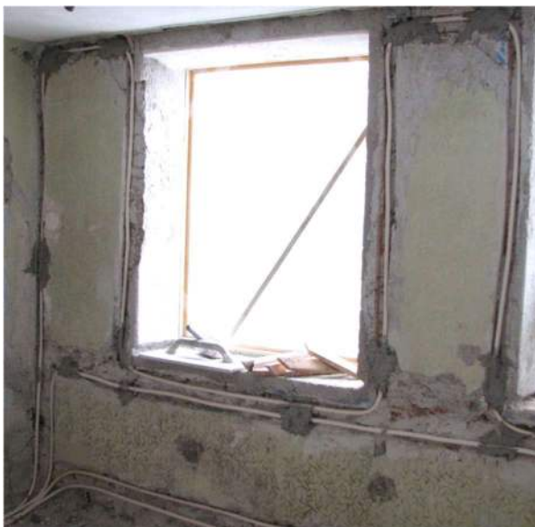
Fig. 18 Refurbishment of the old town centre of Hallein: Installation of copper pipes on the inside of the wall and around the windows @Habersatter Lindner
