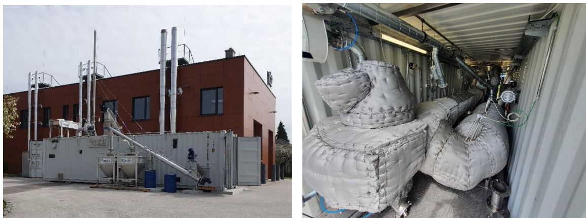
Figure 8: left: Pilot Scale pyrolysis plant from outside; right: pyrolysis plant inside container, pyrolysis reactor on left and gas burner on right side
