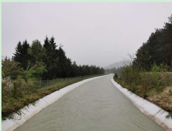
Figure 14: Fenced outlet to power plant at river Gail is a significant barrier.
