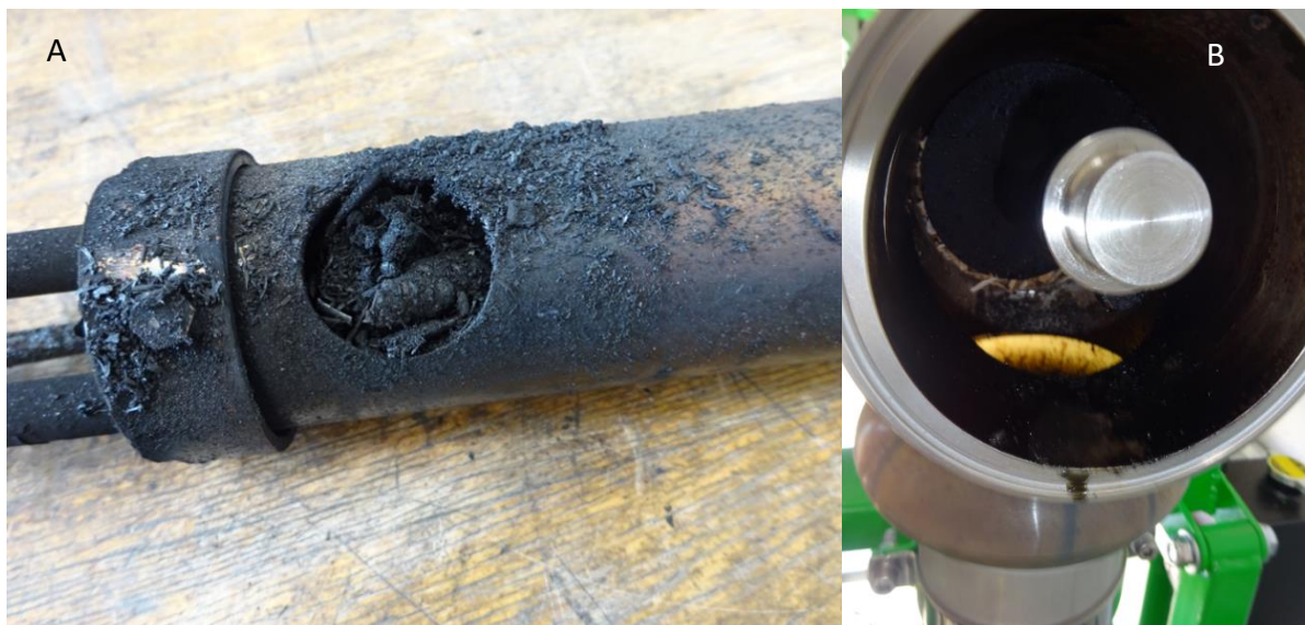
Figure 7: A) Picture of the gas outlet located in the hot reactor core. It can be clearly seen that the exit for the syngas is blocked by biochar particles. B) Exemplary picture of the tar deposition issue, located at the feeding screw
